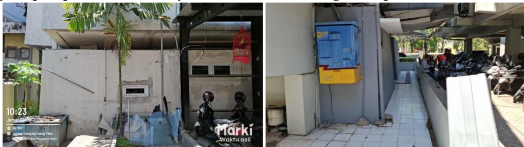
Figure 2. Ground Water Tank (GWT), Water Pump, and Electrical Panel
