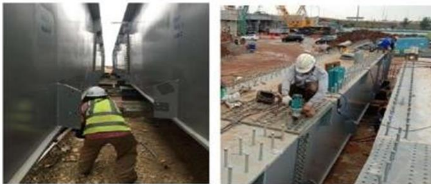
Figure 4. Adjusting the chamber and tightening the segment join bolts Source: Wika-Nindya KSO Implementation RKK Document
